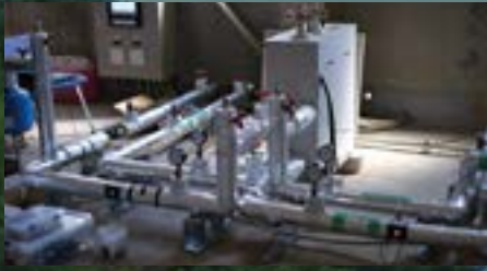
The geothermal heat pump experimental system
